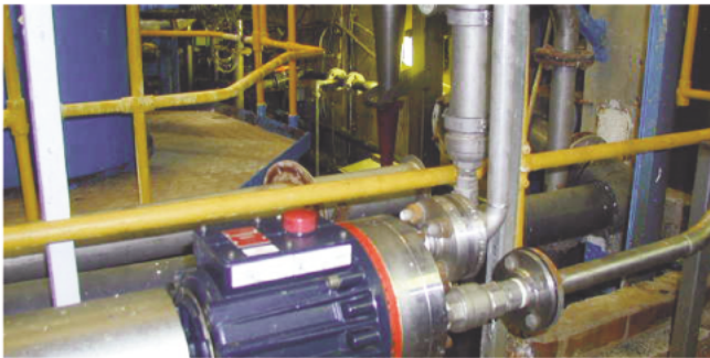
Figure 4: G25 pump on paper machine at Simpson-Clough Mill
